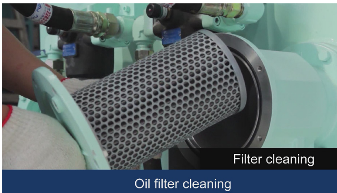
Oil filter cleaning
