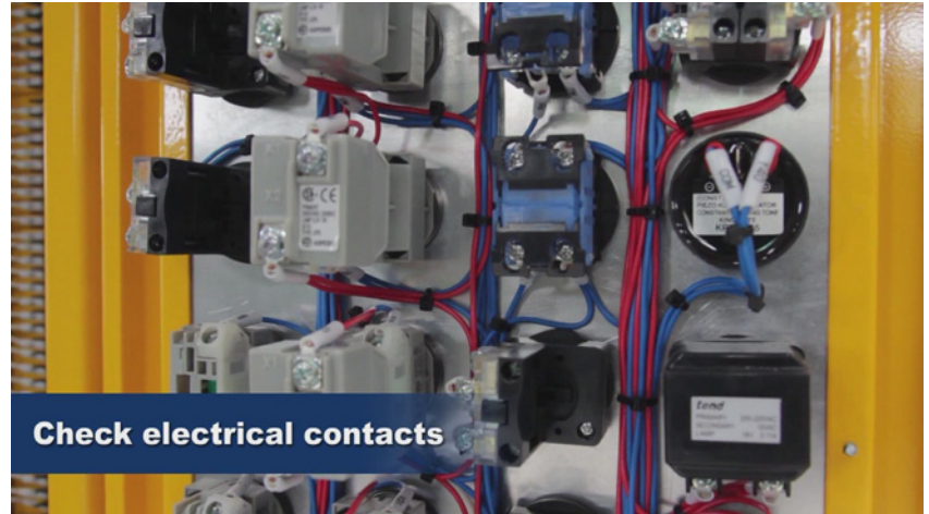
Checking electric poing
